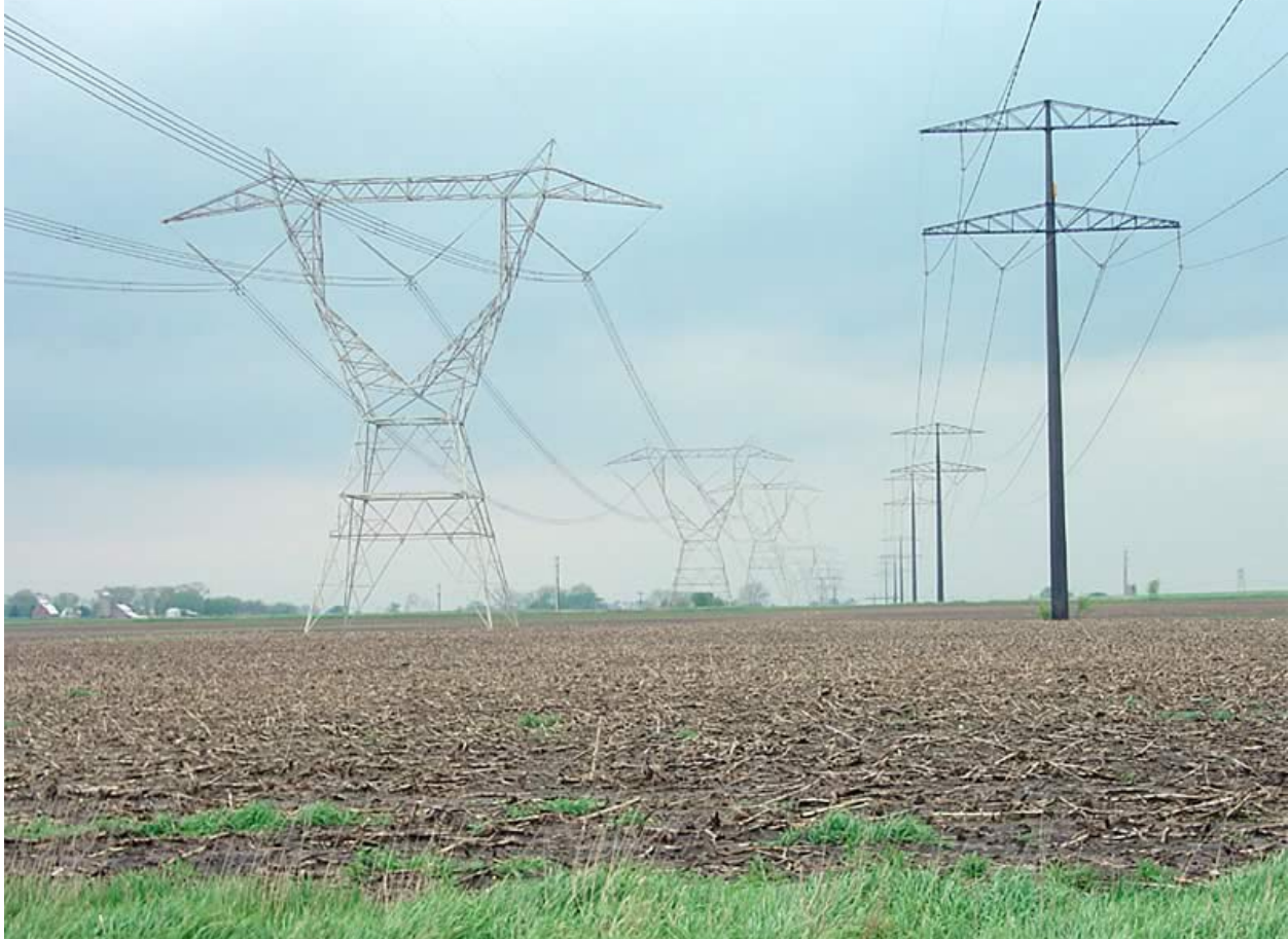
1 2 FIGURE 5.12-1 Transmission Towers: Lattice (left) and Monopole (right) (Source: Argonne 2007)
