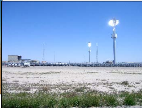
5 MW Power Tower Plant Lancaster, CA
