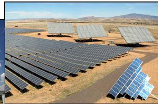
PV Plant Prescott, AZ
